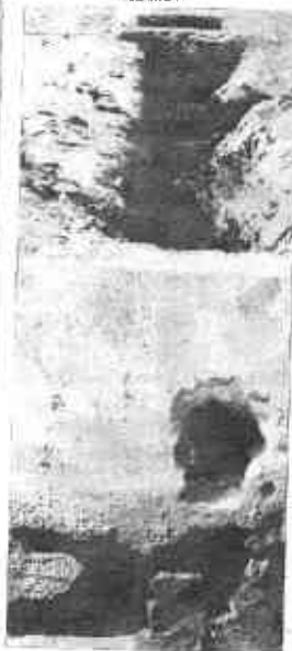
Drain corroded due to toxic discharge from an industry. Photograph: Farhan Anwar.
